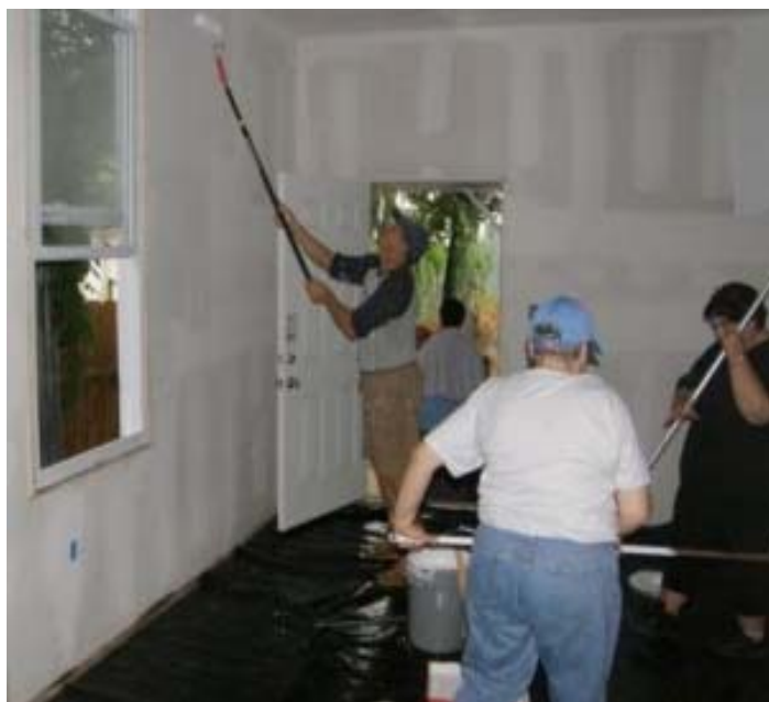
Delaware Valley Rotary Volunteers George Merz, Isabel Lally, and Tish Mayo work on repairing and painting the inside of a home which was damaged by Hurricane Katrina in New Orleans in October.
